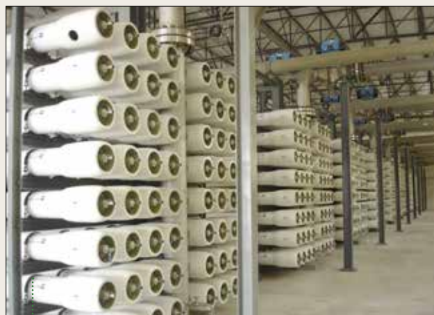
Areva Desalination Plant
