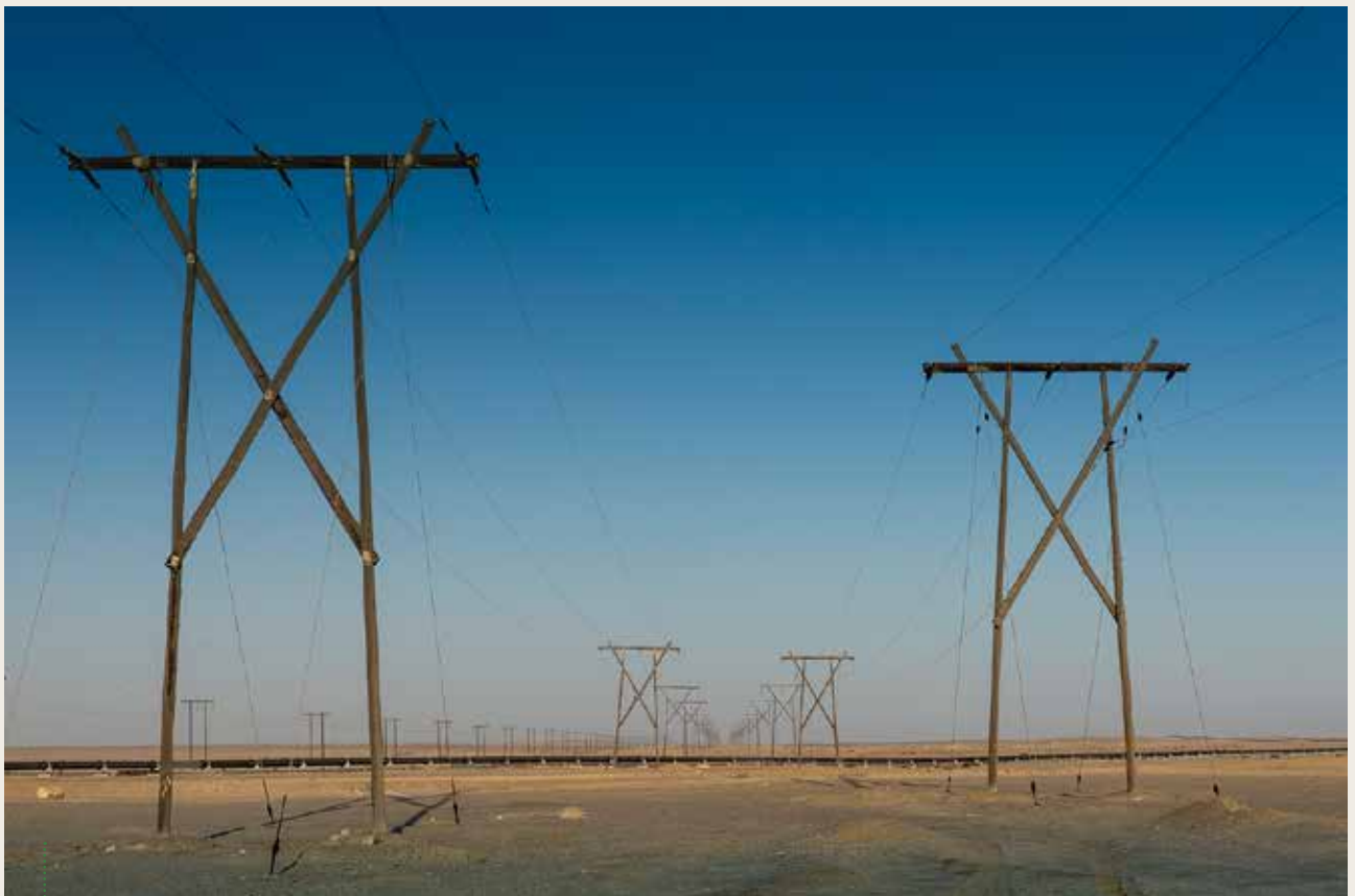
Electrical transmission lines
