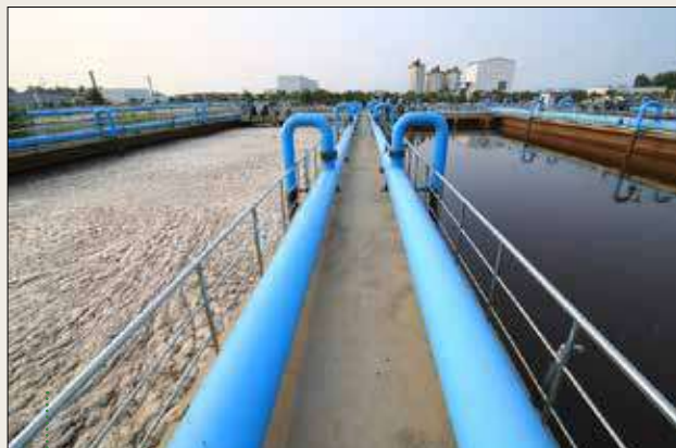
End-of-pipe treatment – wastewater treatment plant to treat pathogens, nutrients and chemicals contained in municipal effluent
