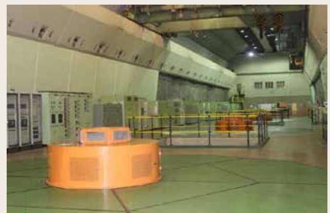
Underground machine hall at Ruacana
