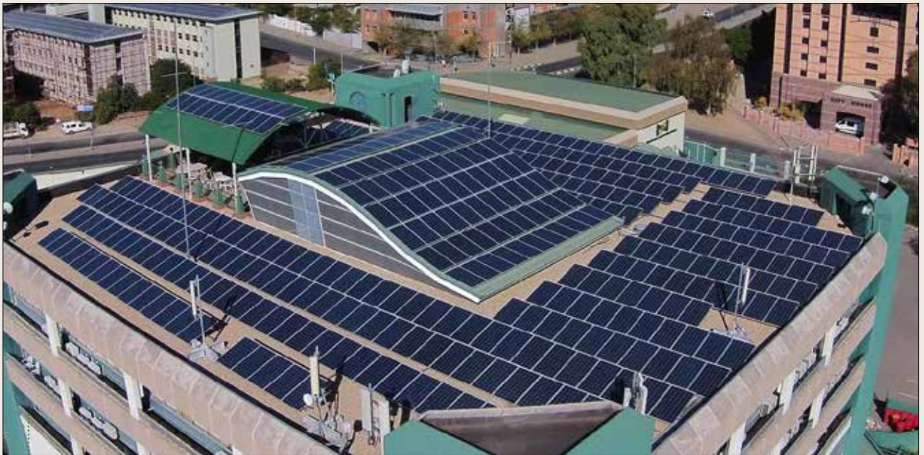
Rooftop solar installation at NamPower
