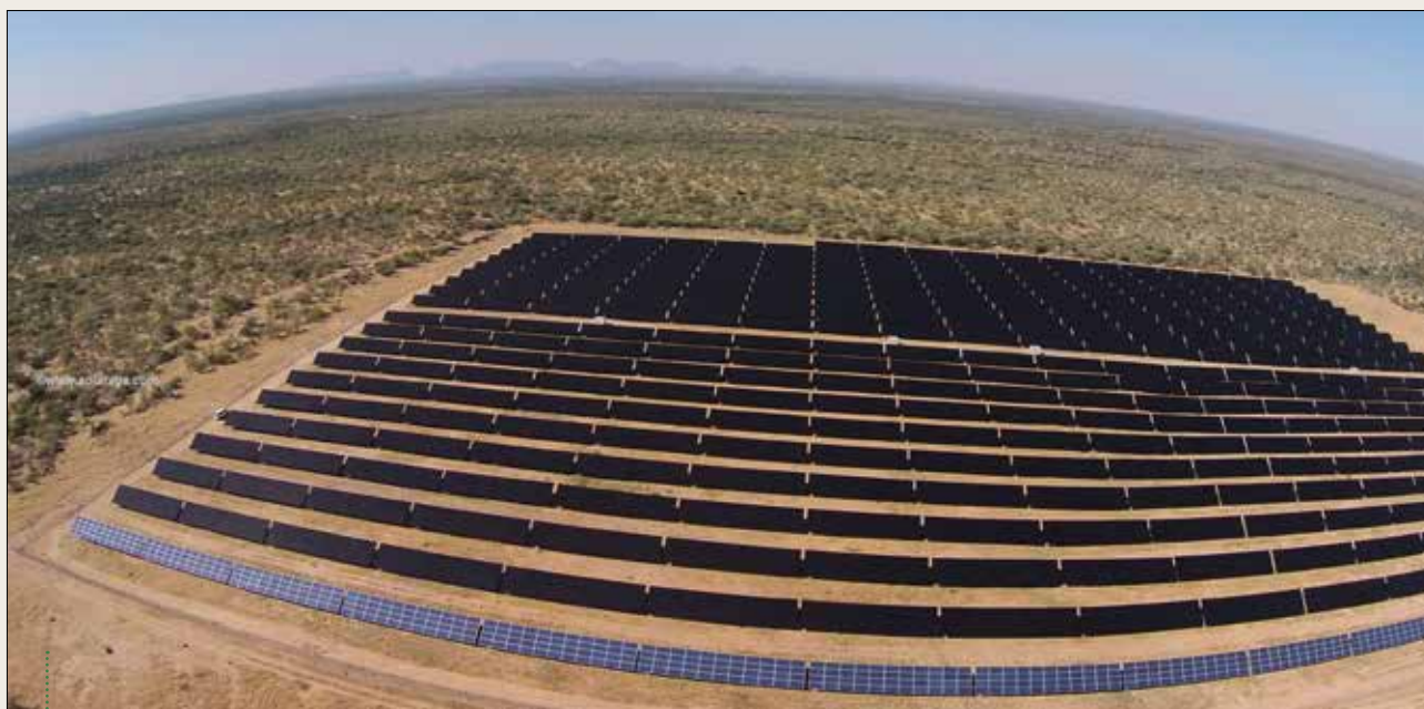
Omburu Photovoltaic Plant
