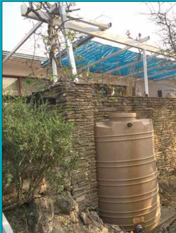
Rainwater harvesting from roof
